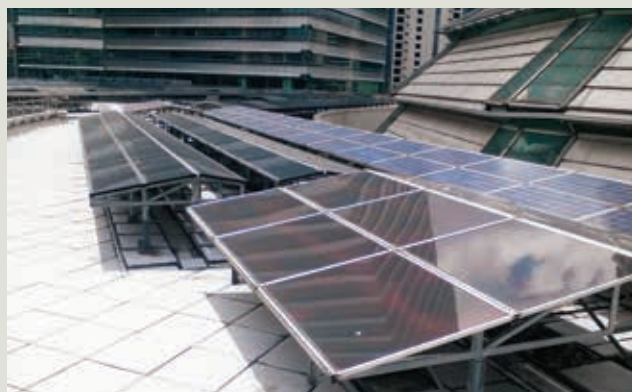
Solar Panel on Suria KLCC rooftop
